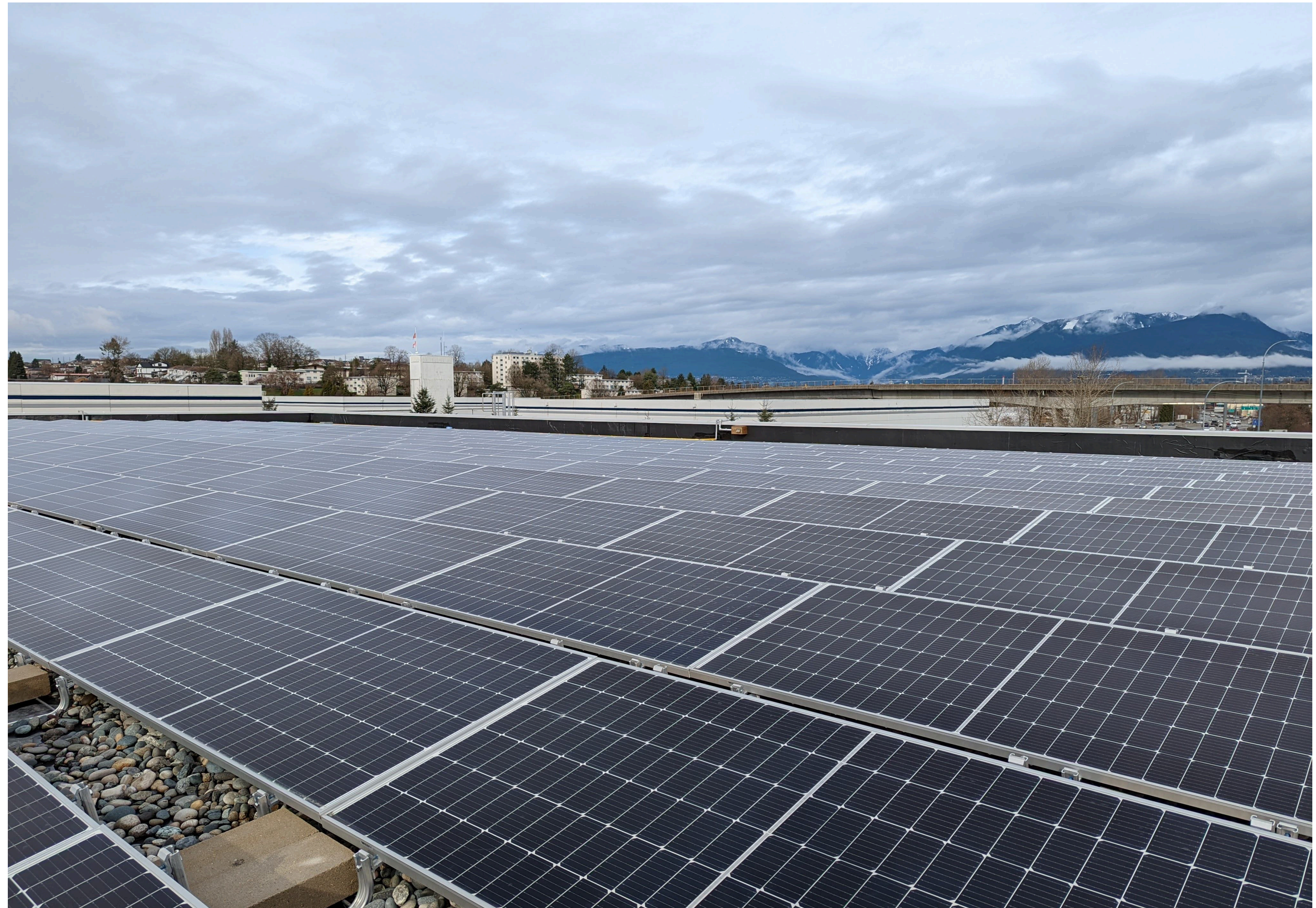
Solar array at Vancouver Film Studios
